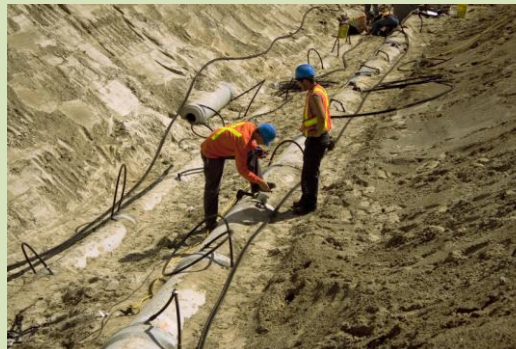
The illustration above shows the installation of the @Source-Energy Pipes in a new subdivision in Sudbury, Ontario in 2009.
